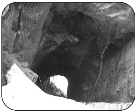
SNOW BLOCKED WEST ENTRANCE TO NEEDLES EYE TUNNEL
